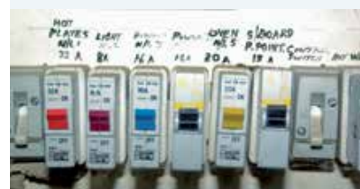
Circuit breakers within a meter box
