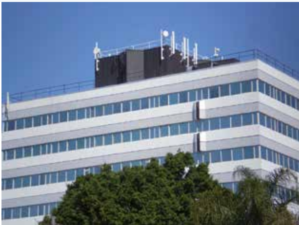
Typical mobile phone base stations
