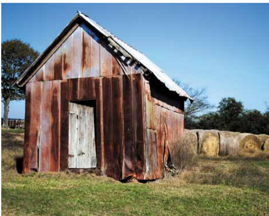
The rusting of this shed is an example of corrosion.
