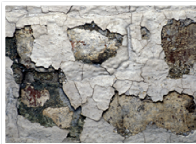
Fig 4.5.12 Flaking from old lead-based paints has been linked to lead poisoning in humans.
