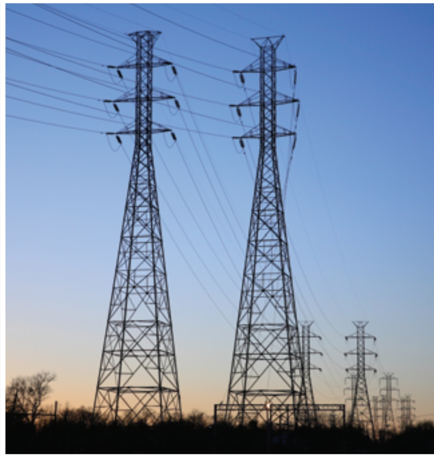
Fig 7.1.2 Electricity is transmitted over long distances as high voltage, low current AC electricity. Electricity is easier to transmit as AC than DC and less energy is lost in the transmission.
